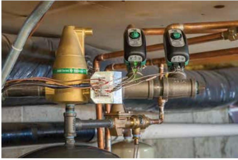
WHAT YOU'LL NEED: Mercier's recipe includes two Taco Zone Sentry zone valves and a 4900 air separator used for the system supply header.
